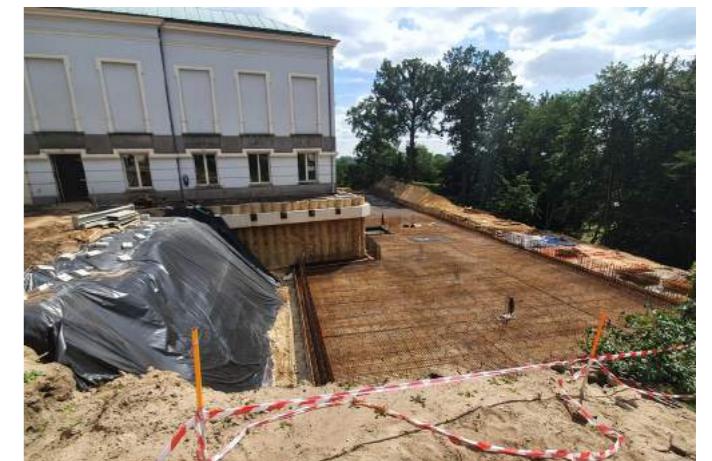
▲ FIGURE 24: CONSTRUCTION SITE WITH PILE WALL AROUND THE HEAD OF THE EXISTING WING
